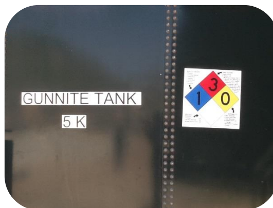
Tanks Signage and Paint
