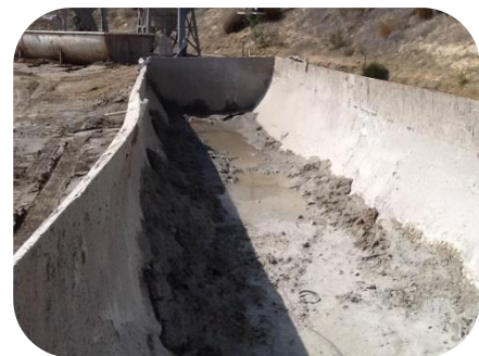
Waste De-Water Bin
