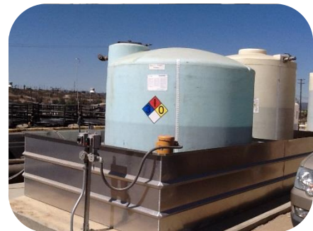
Tank Secondary Containment
