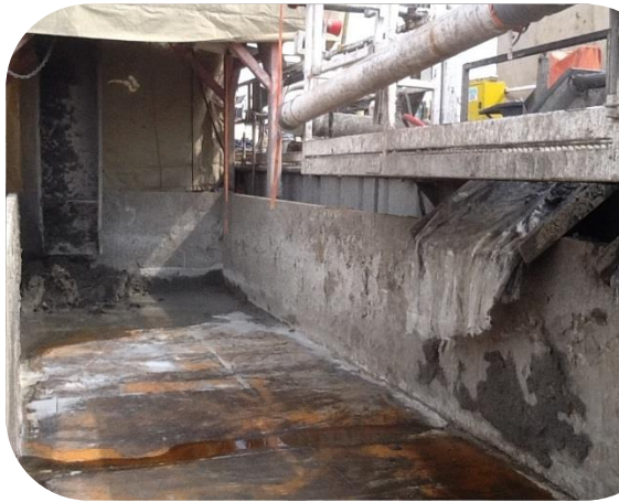
Drill Mud Bin
