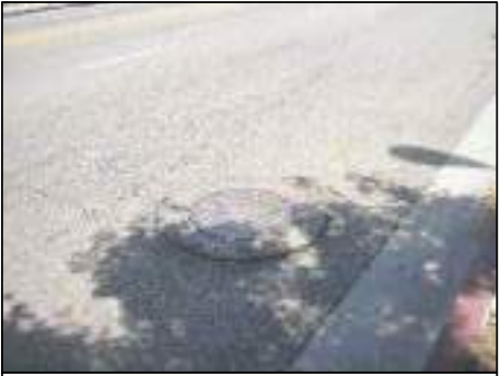
EXISTING MANHOLE PROTRUDES FROM PAVEMENT. ADJUST TO GRADE.
