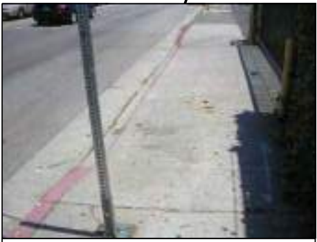
RECONSTRUCT DRIVEWAY TO MEET ADA REQUIREMENTS.
