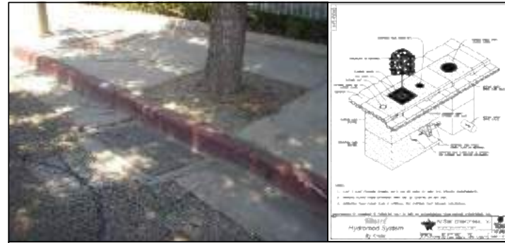
DAMAGED GRATE INLET CATCH BASIN. OPPORTUNITY TO RECONSTRUCT CATCH BASIN WITH ADJACENT STORM WATER BIO-RETENTION FILTRATION SYSTEM (LID)
