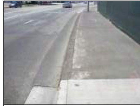
ALL CURB/GUTTER AND SIDEWALK IS TO BE REPLACED IN CONJUNCTION MIXED-USED DEVELOPMENT AT 8770 WASHINGTON BOULEVARD.
