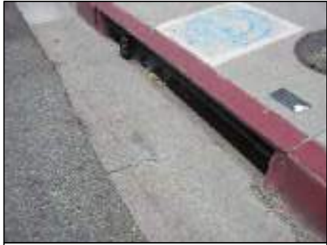
EX. CATCH BASIN. INSTALL CITY APPROVED CATCH BASIN SCREEN AND/OR DEBRIS COLLECTOR (BMP).
