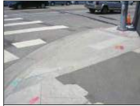
FUTURE CURB RETURN AND ADA CURB RAMP PER TRAFFIC IMPACT ANALYSIS REPORT (JULY 2010) FOR 8770 WASHINGTON BOULEVARD MIXED-USE DEVELOPMENT.
