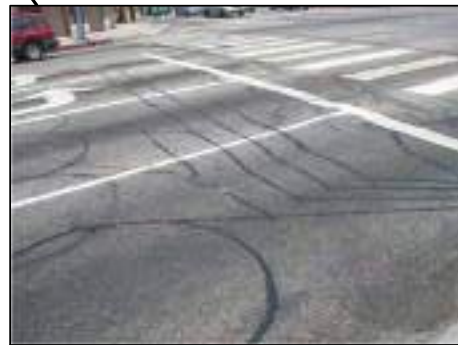
REPAIR DAMAGED AC PAVEMENT. RE-CUT DETECTOR LOOPS IF NECESSARY.
