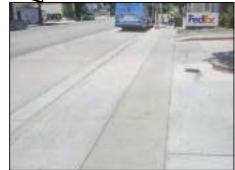
EXISTING DRIVEWAY HAS 3' PEDESTRIAN PATH. RECOMMEND RECONSTRUCTION OF DRIVEWAY WITH A MINIMUM 4' PEDESTRIAN PATH.
