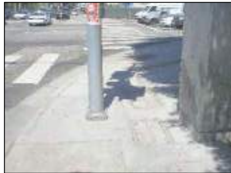
EXISTING 3' CLEARANCE BETWEEN TRAFFIC SIGNAL POLE AND CONTROLLER CABINET. RECOMMENDED TRAFFIC SIGNAL MODIFICATION TO INCREASE CLEARANCE.
