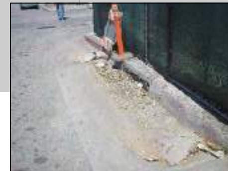
FUTURE RECONSTRUCTED CATCH BASIN. INSTALL CITY APPROVED CATCH BASIN SCREEN AND/OR DEBRIS COLLECTOR (BMP).
