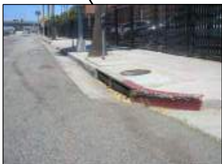
EX. CATCH BASIN. OPPORTUNITY TO REMOVE ADJACENT TREE & REPLACE WITH STORM WATER BIORETENTION FILTRATION SYSTEM/TREE WELL (LID)
