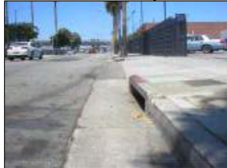
EX. CATCH BASIN. INSTALL CITY APPROVED CATCH BASIN SCREEN AND/OR DEBRIS COLLECTOR (BMP). OPPORTUNITY TO REMOVE ADJACENT TREE & REPLACE WITH STORM WATER BIORETENTION FILTRATION SYSTEM/TREE WELL (LID)
