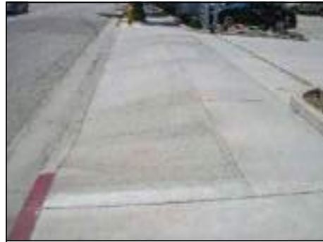
EXISTING DRIVEWAY IS AT 19.5% WHICH EXCEEDS CURRENT STANDARDS. RECOMMEND RECONSTRUCT DRIVEWAY.
