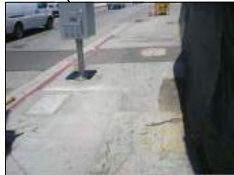
CURB/GUTTER, SIDEWALK, AND CURB RAMPS ARE TO BE RECONSTRUCTED AS PART OF THE EXPOSITION METRO LIGHT RAIL PROJECT.
