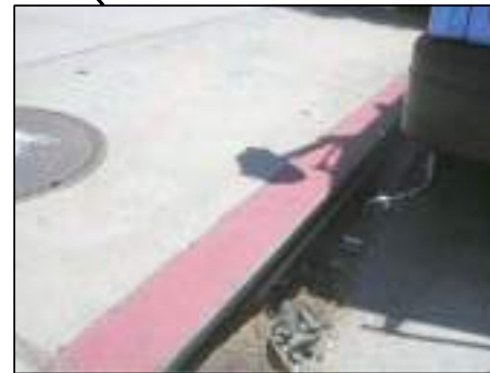
EX. CATCH BASIN. INSTALL CITY APPROVED CATCH BASIN SCREEN AND/OR DEBRIS COLLECTOR (BMP).
