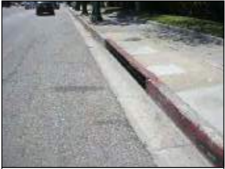
EX. CATCH BASIN. INSTALL CITY APPROVED CATCH BASIN SCREEN AND/OR DEBRIS COLLECTOR (BMP).
