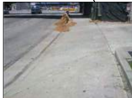
EXISTING DRIVEWAY DOES NOT MEET ADA REQUIREMENTS. RECOMMEND RECONSTRUCTION OF DRIVEWAY TO MEET CURRENT STANDARDS
