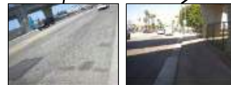
DAMAGED/TEMPORARY PAVEMENT/SIDEWALK. REMOVE AND REPLACE.
