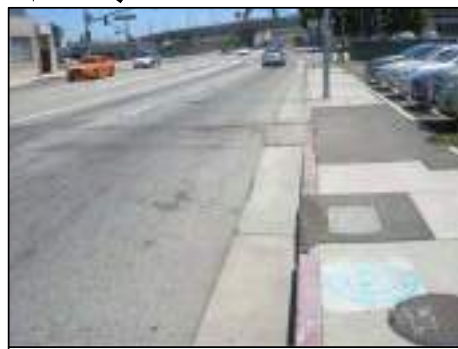
REMOVE RAIL ROAD TRACK COMPLETE, RECONSTRUCT ROADWAY, CURB, GUTTER, AND SIDEWALK AS NEEDED.
