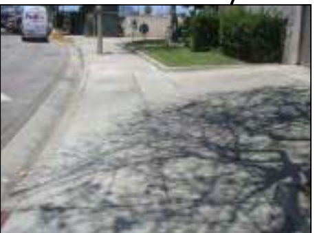
EXISTING DRIVEWAY HAS 3' PEDESTRIAN PATH. RECOMMEND RECONSTRUCTION OF DRIVEWAY WITH A MINIMUM 4' PEDESTRIAN PATH.
