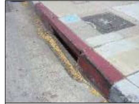
EX. CATCH BASIN. INSTALL CITY APPROVED CATCH BASIN SCREEN AND/OR DEBRIS COLLECTOR (BMP).
