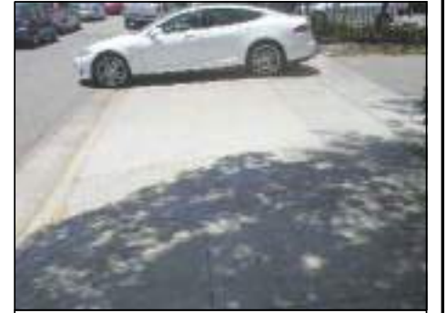
PEDESTRIAN PATH AT BACK OF DRIVEWAY IS 3'. RECOMMEND TO RECONSTRUCT DRIVEWAY TO ACCOMPLISH A 4' MINIMUM PEDESRIAN PATH AT 2%.
