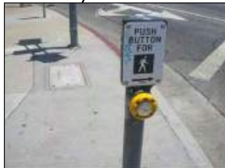
RECOMMEND TO UPGRADE ALL PEDESTRIAN PUSH BUTTONS TO CITY APPROVED APS UNITS. TYPICAL FOR ALL PPB'S AT THIS INTERSECTION.
